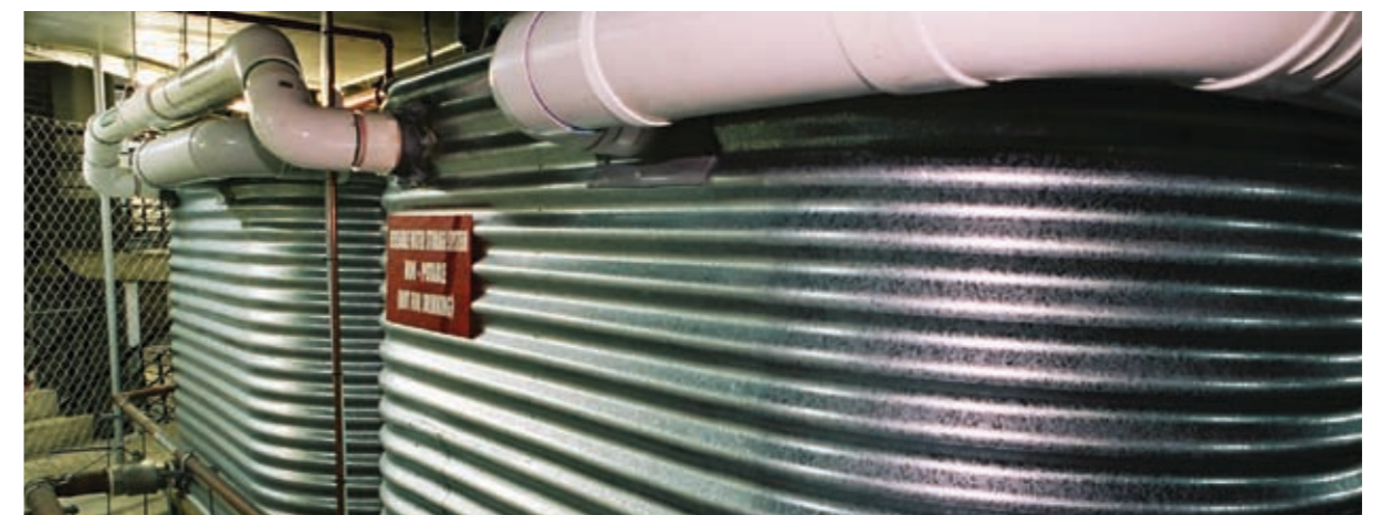
Photograph 10 – Rainwater captured in tanks at Investa's 73 Miller Street building in North Sydney, is used to irrigate gardens on the building's rooftop and balconies.
